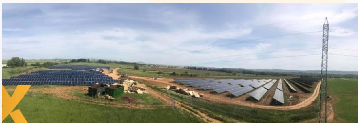
Photovoltaic plant of Cañamares in Guadalajara
