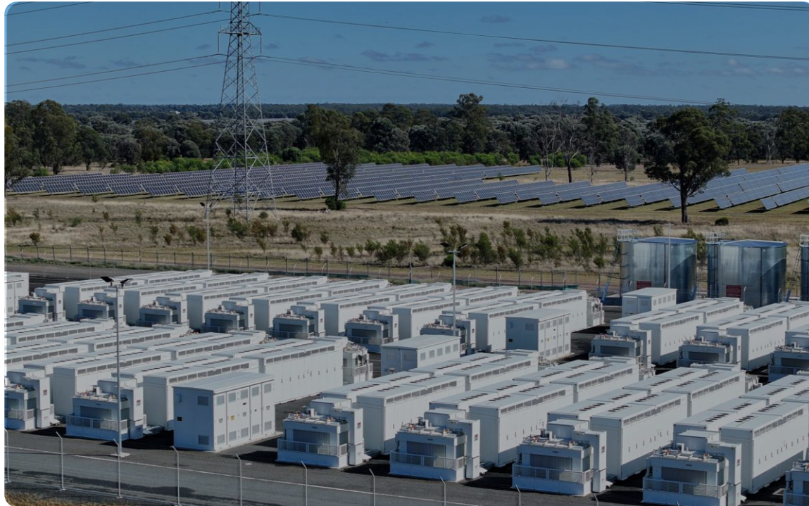
Western Downs Battery, Queensland, Australia
