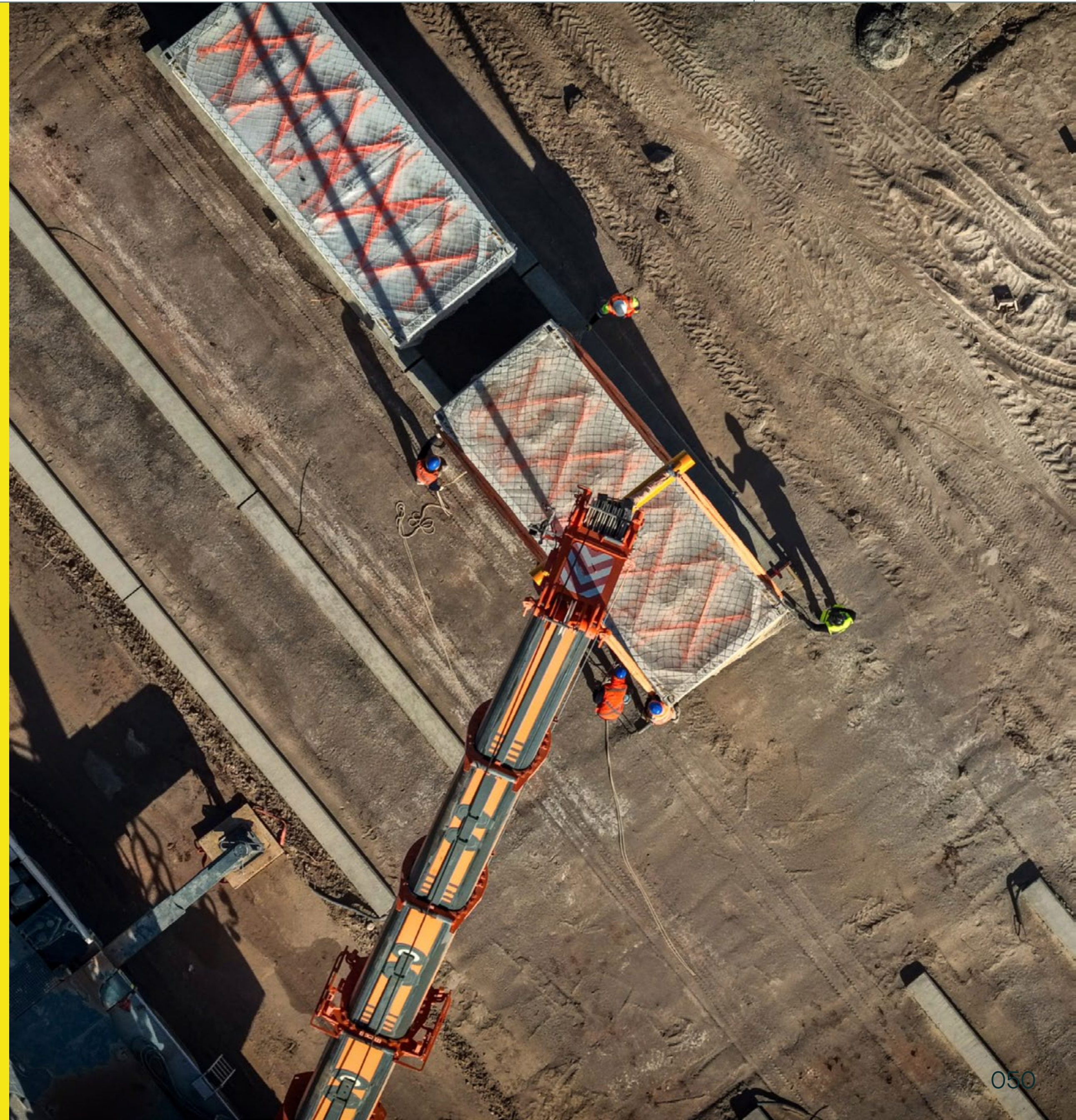
Elena 446 MW + 3.5 GWh hybrid plant, Chile
