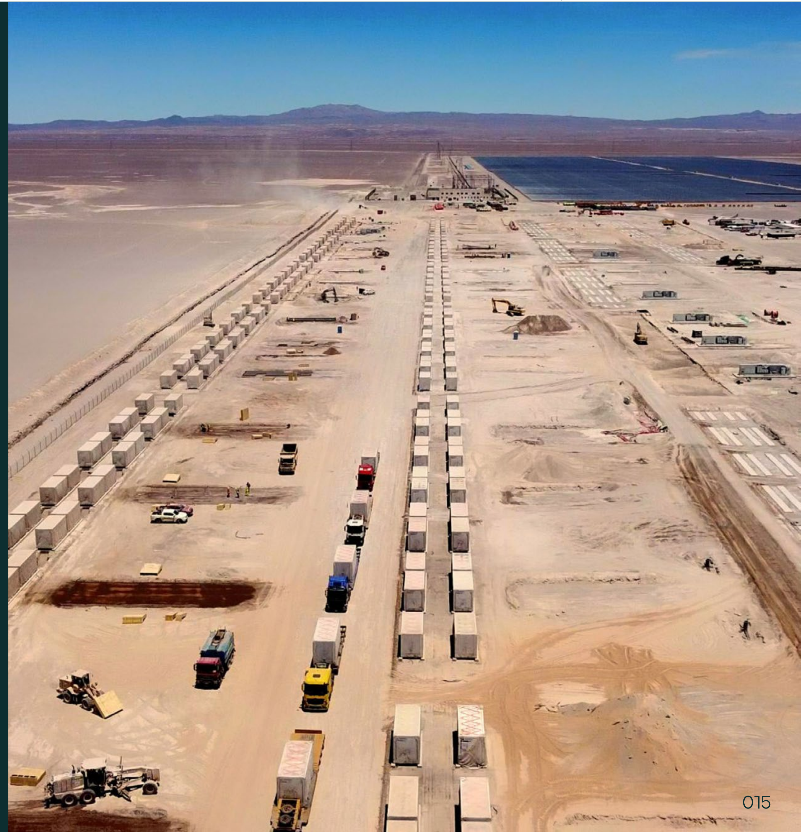
Elena 446 MW + 3.5 GWh hybrid plant, Chile
