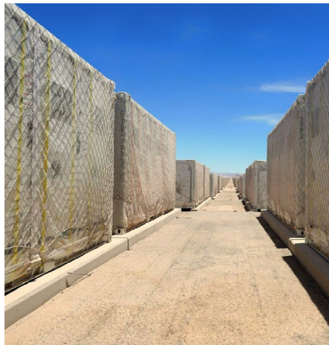
Elena 446 MW + 3.5 GWh hybrid plant, Chile
