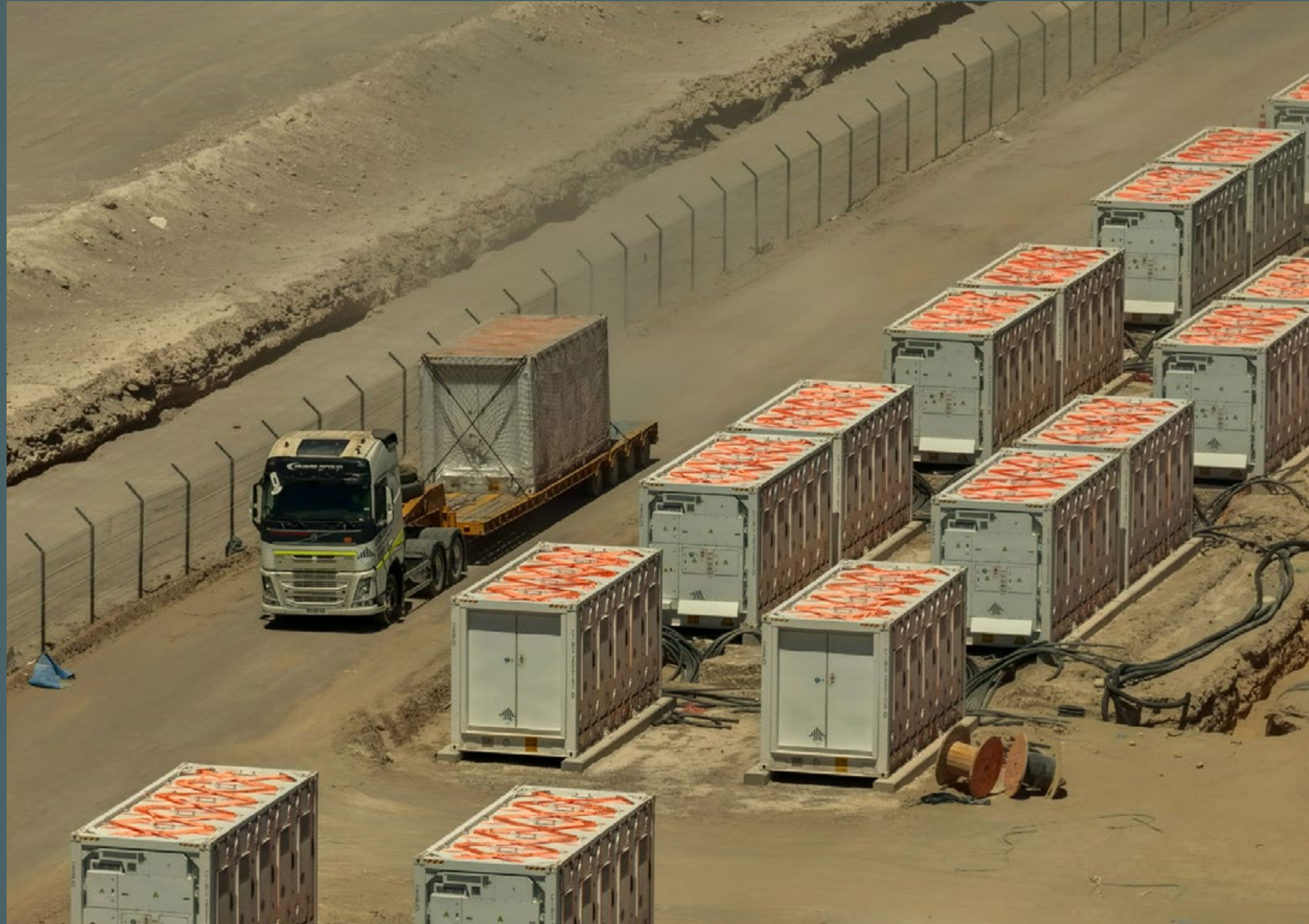
Elena 446 MW + 3.5 GWh hybrid plant, Chile
