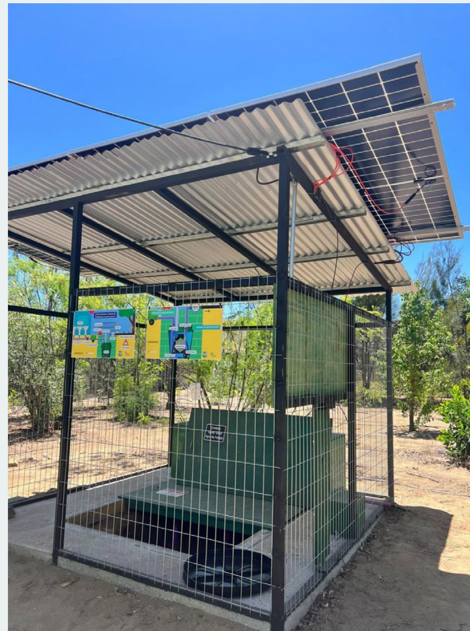
Solar panel-powered pump
