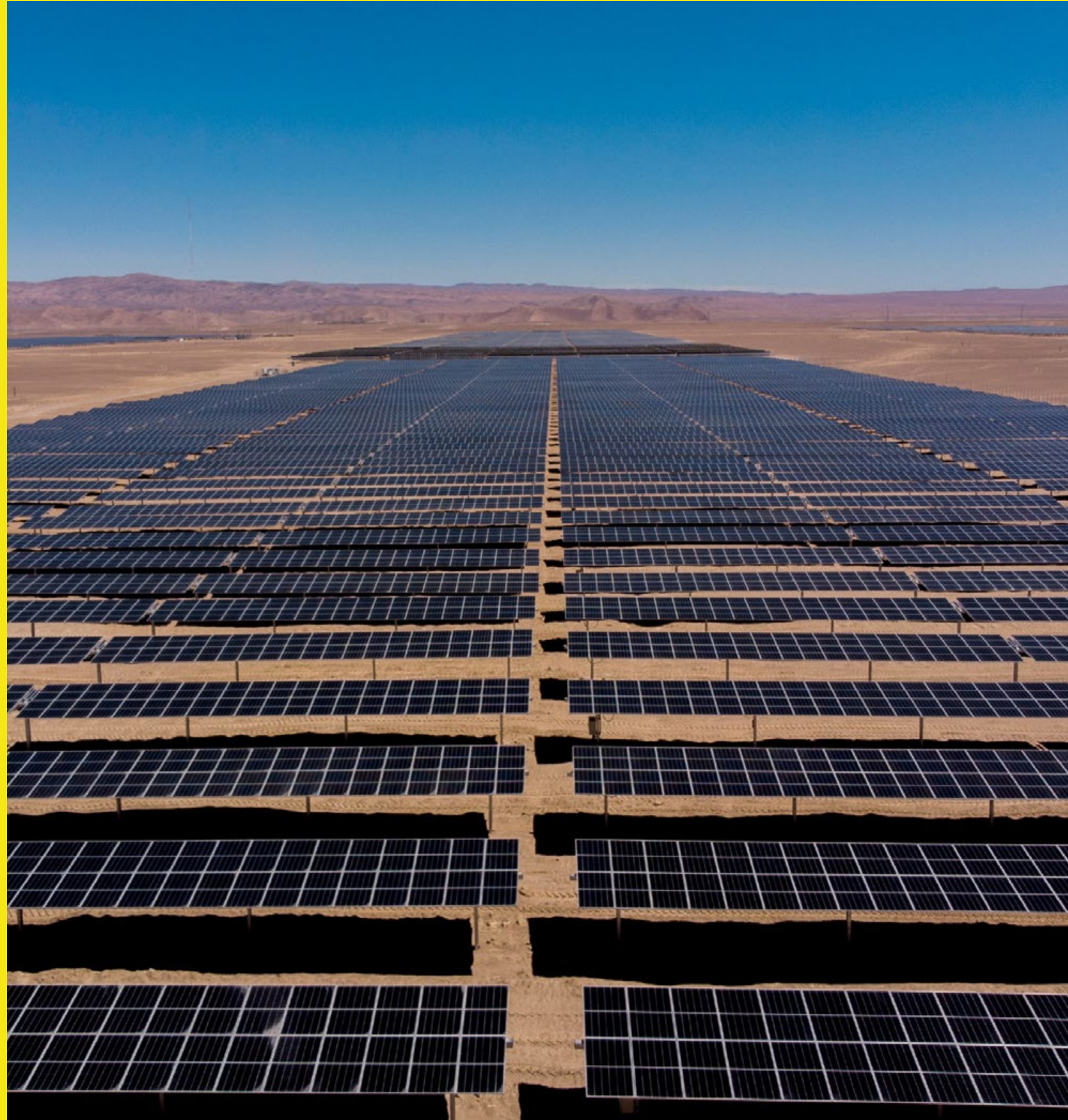
Quillagua 103 MW PV plant, Chile
