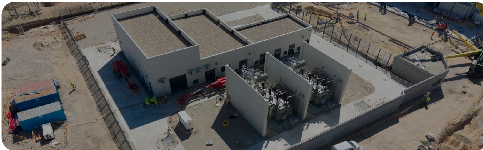
Alcalá Data Center, Madrid, Spain
