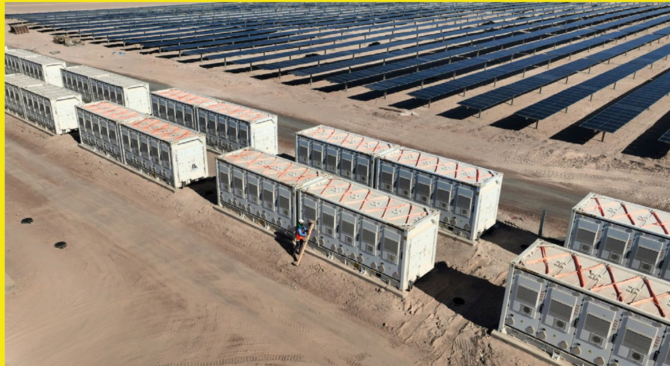
Elena 446 MW + 3.5 GWh hybrid plant, Chile
