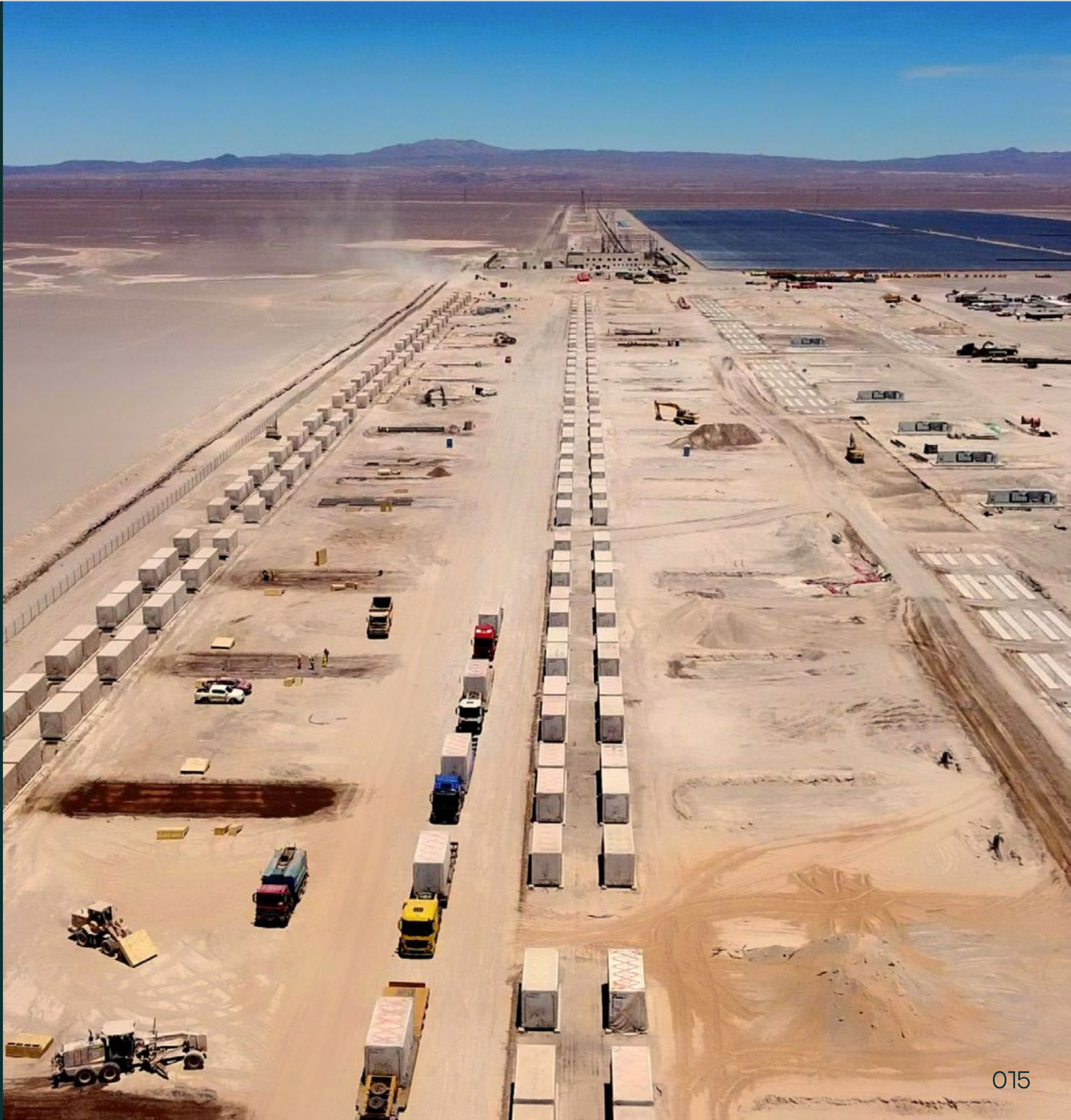
Elena 446 MW + 3.5 GWh hybrid plant, Chile
