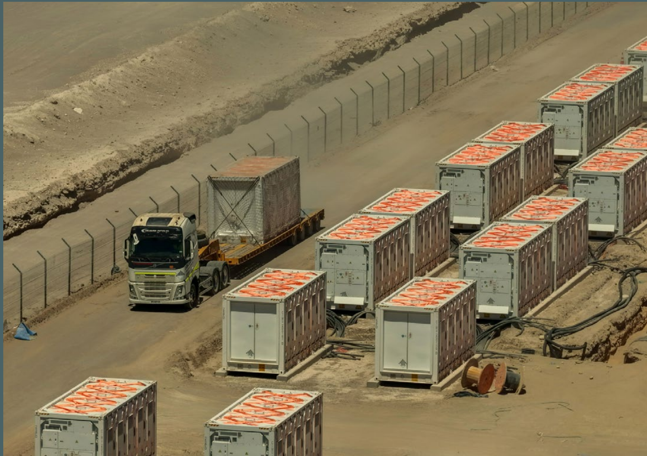
Elena 446 MW + 3.5 GWh hybrid plant, Chile
