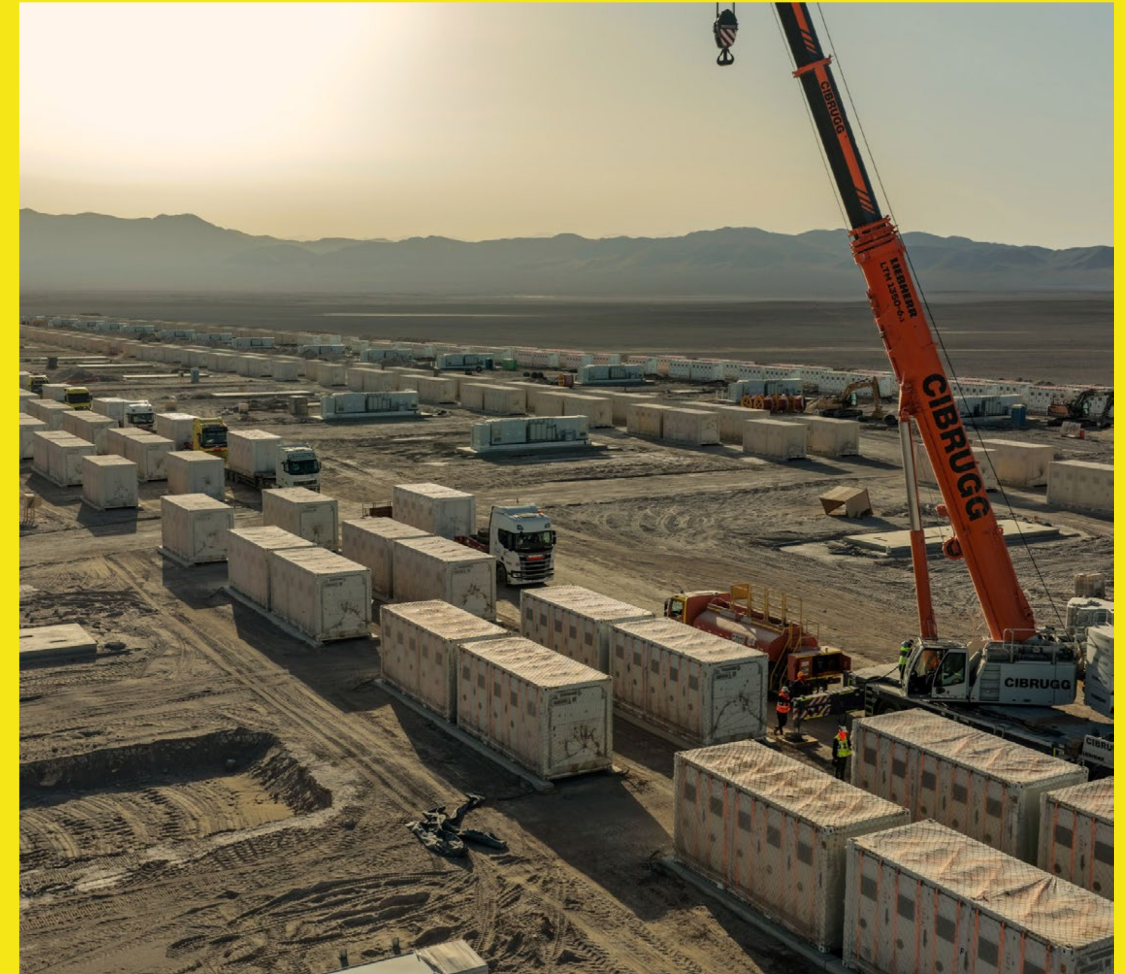
Elena 446 MW + 3.5 GWh hybrid plant, Chile
