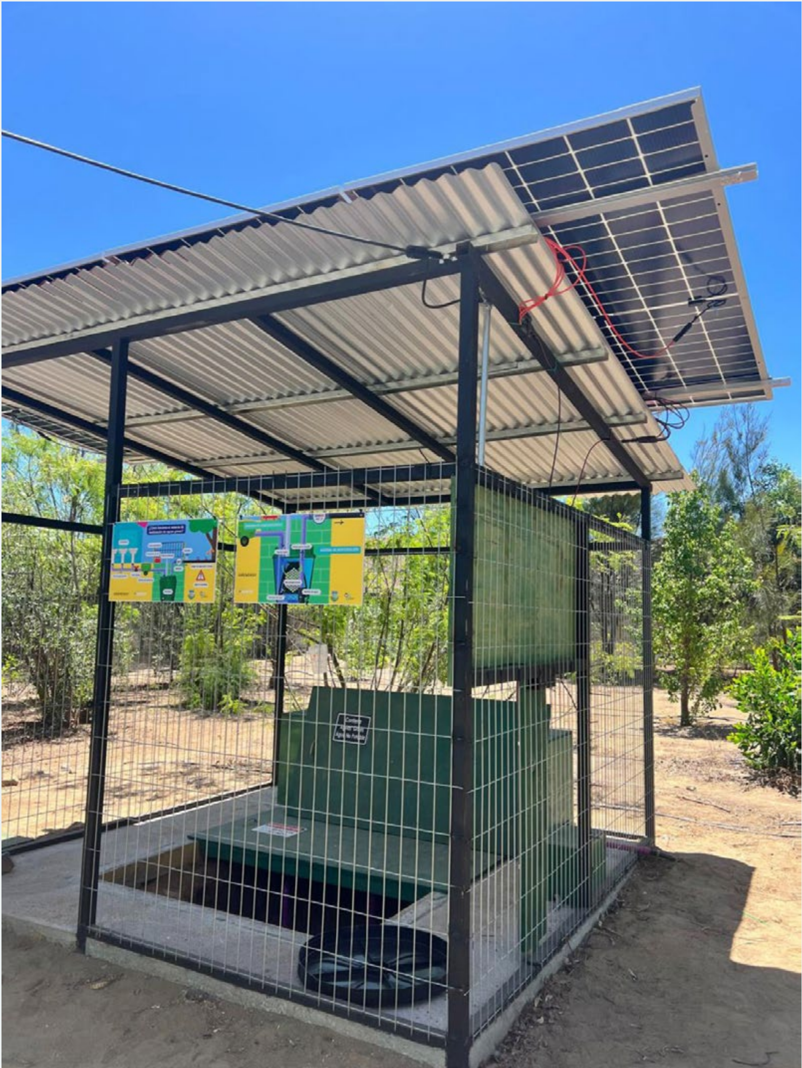
Solar panel-powered pump
