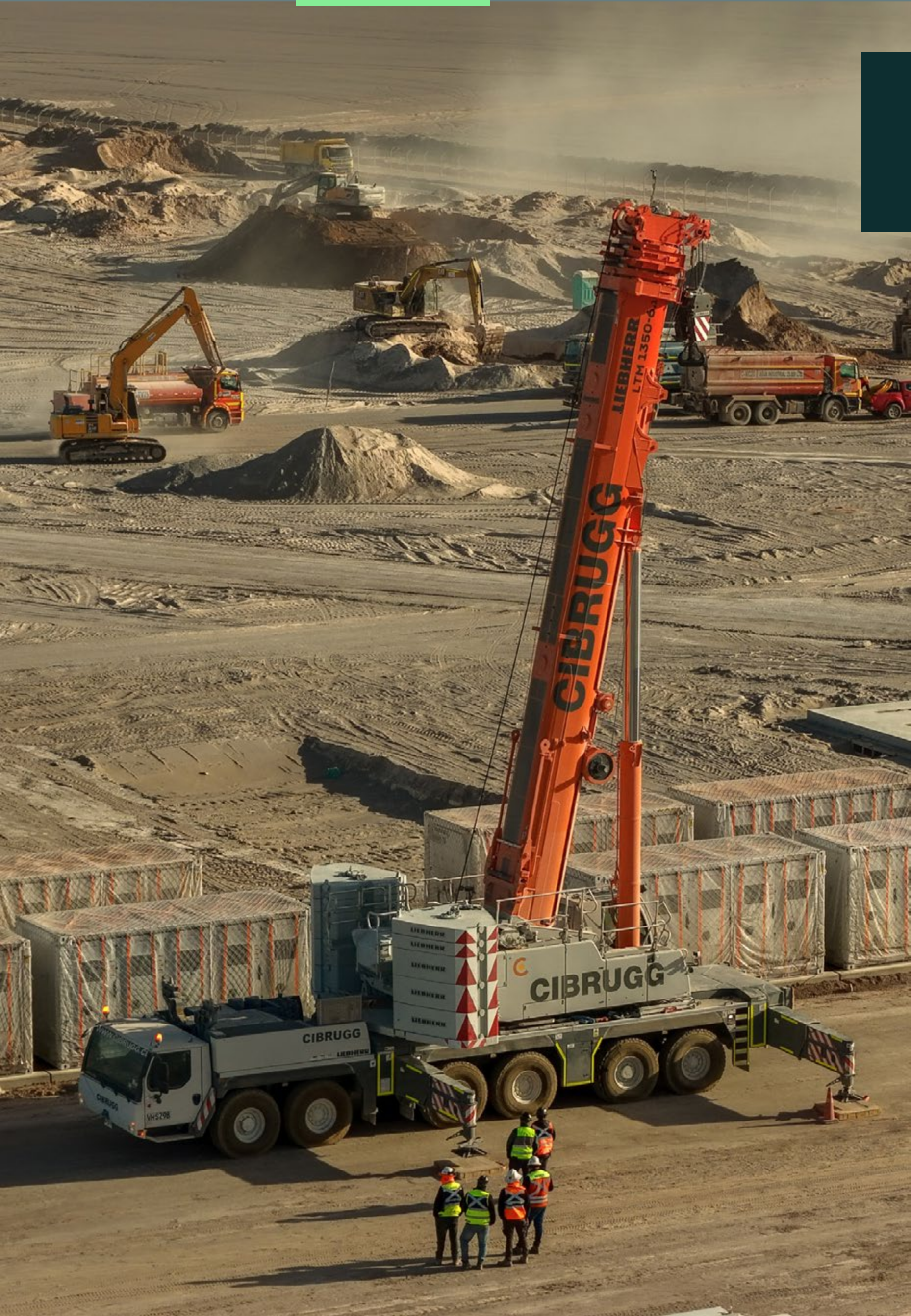
Elena 446 MW + 3.5 GWh hybrid plant, Chile
