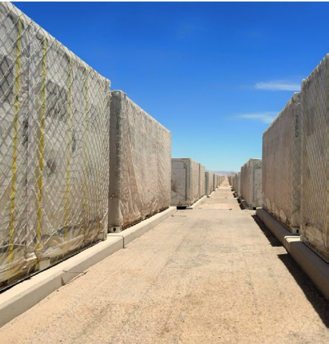
Elena 446 MW + 3,5 GWh hybrid plant, Chile
